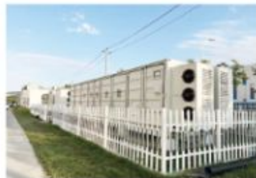
3MW/6MWh, C&amp;I ES project, China
