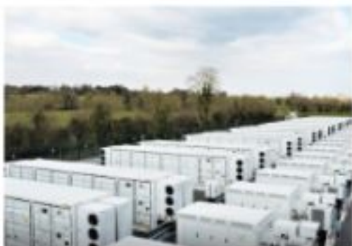
70MW/340MWh, frequency regulation, Italy
