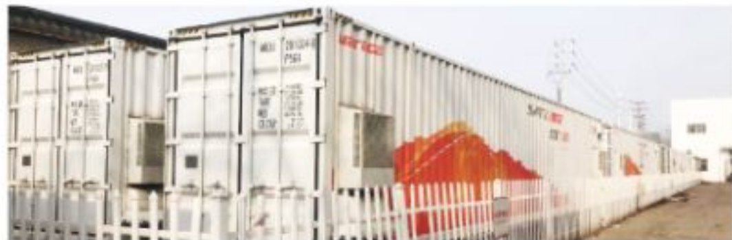
7MW/30MWh, C&amp;I ES project, Jiangsu, China
