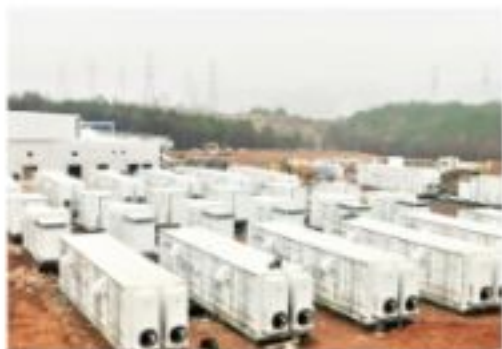
100MW/200MWh, frequency regulation, Hunan, China
