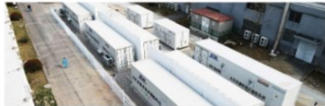
3.75MW/15MWh, C&amp;I ES project, China
