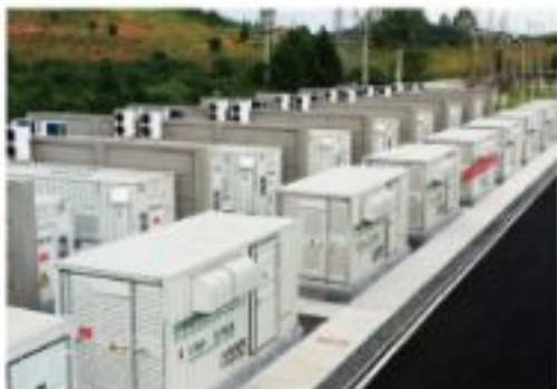
74MW/108MWh, frequency regulation, Hunan, China
