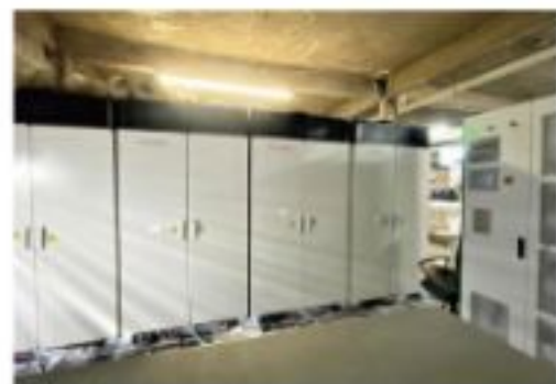
Outdoor Cabinet ES Project, Mexico
