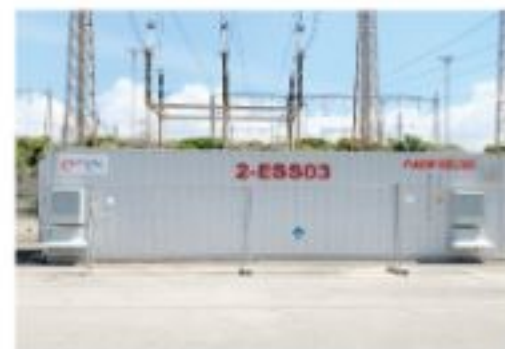
22MW/22MWh, thermal plant AGC frequency regulation, Italy
