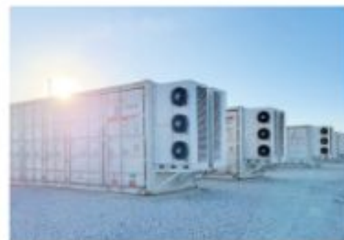
71MW/130MWh, wind+ESS, Texas, USA
