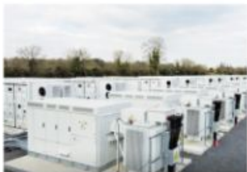
50MW/32.44MWh, frequency regulation, Ireland
