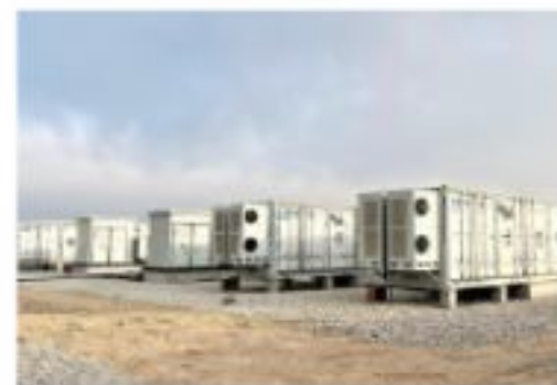
60MW/125MWh, PV+ESS, Xinjiang, China
