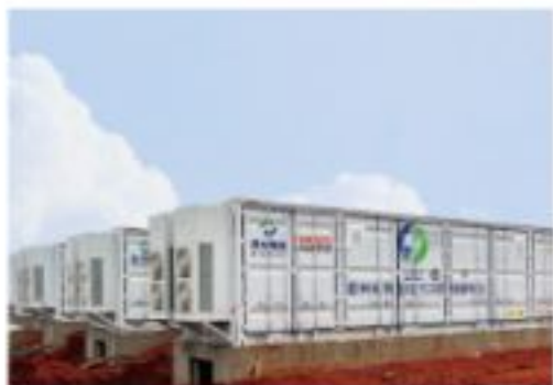
200MW/400MWh, frequency regulation, Guangdong, China
