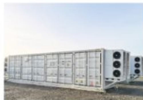
40MW/55MWh, PV+ESS, USA
