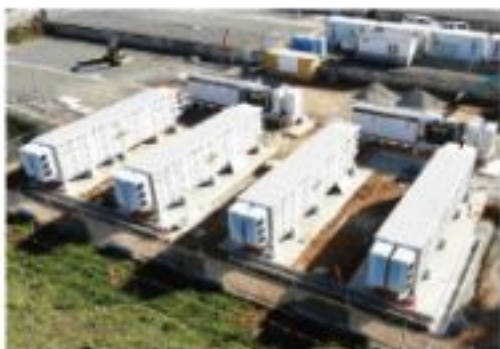
10MW/20MWh, frequency regulation, Australia
